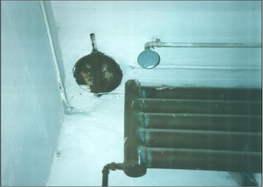
Fig. 11: Ventilation opening, showers and radiator
