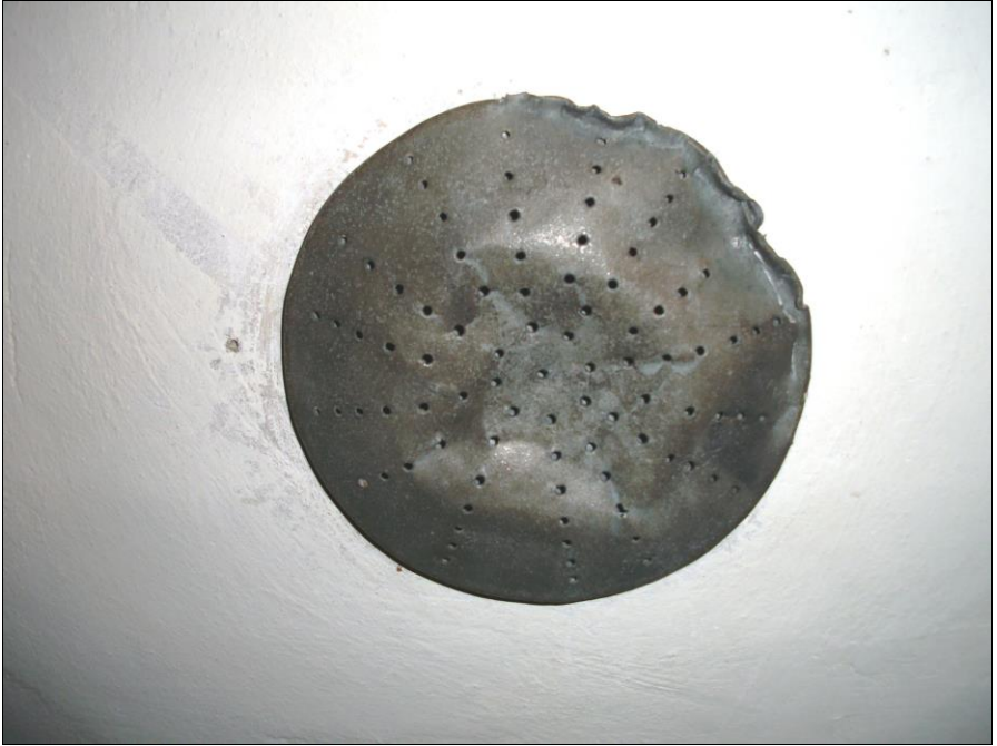
Photo 5: Sole remaining intact head.
