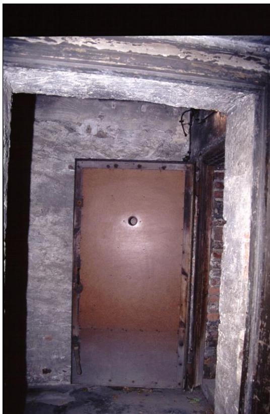
Illustration 4: Make-shift air-raid-shelter door of Krematorium I made of wood with a thin sheet metal cover, probably built by inmates in the camp's workshop.
